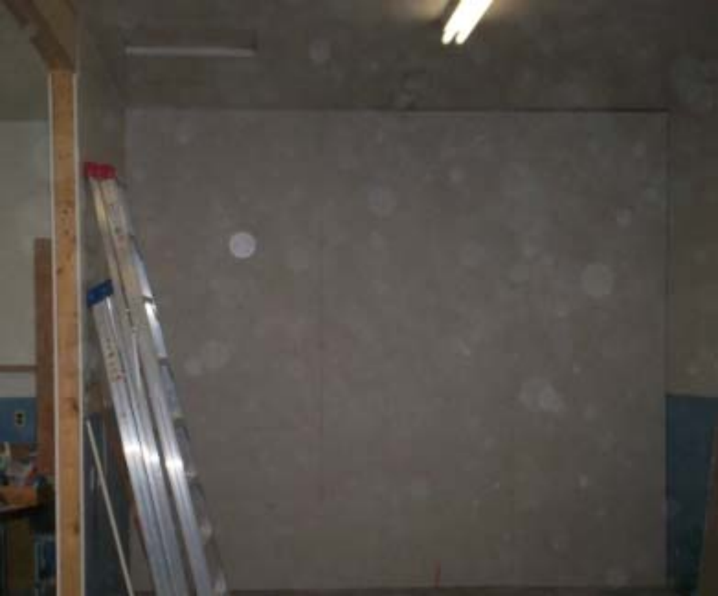
OK, so the finished wall is less than sexy until the paint goes on and that dust got my camera again! Oh, and those ladders keep posing for pictures!
