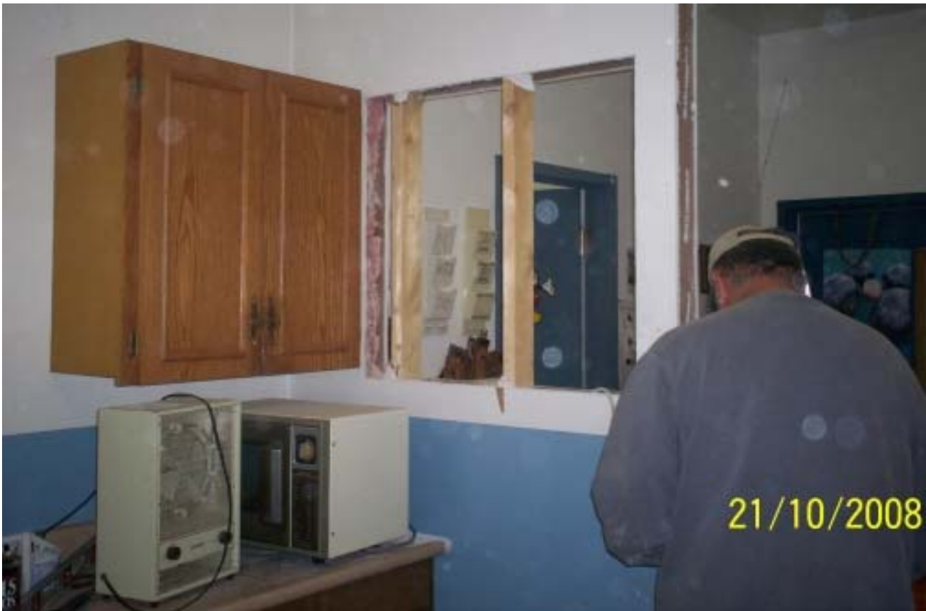
Gradually, kitchen equipment were transferred from the previous area to the new kitchen area and electrical wiring was changed to accommodate.
