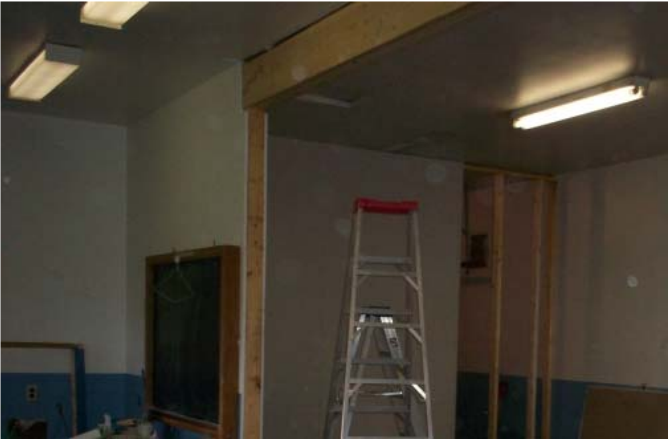
Meanwhile back in the main room, the gyprock goes up on the divider wall and the support beam is added for additional support.
